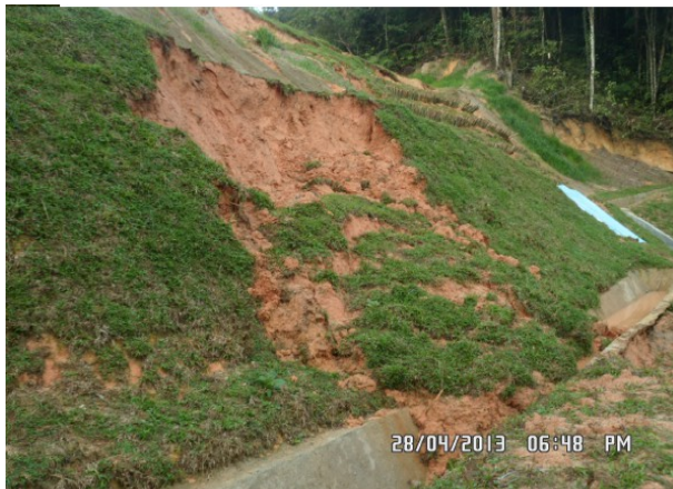
Plate 1: Slope undergoing continous shallow facial failures.
